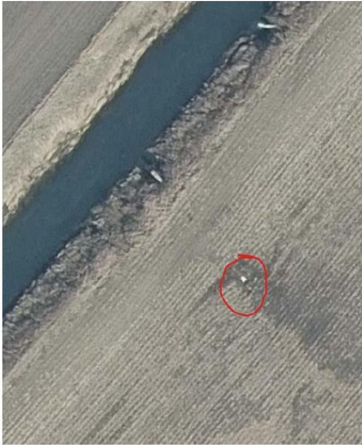
Parcel 3: A culvert in the middle of a cropped field in Piatt County directs runoff directly into a nearby waterway, bypassing a modest non-cropped buffer.
